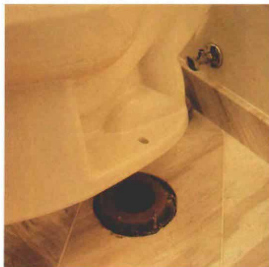
14. The closet flange should end up atop the finished floor surface, but it doesn't always work out that way. In the installation shown here, another wax ring has been added to the gasket to make up the difference.
