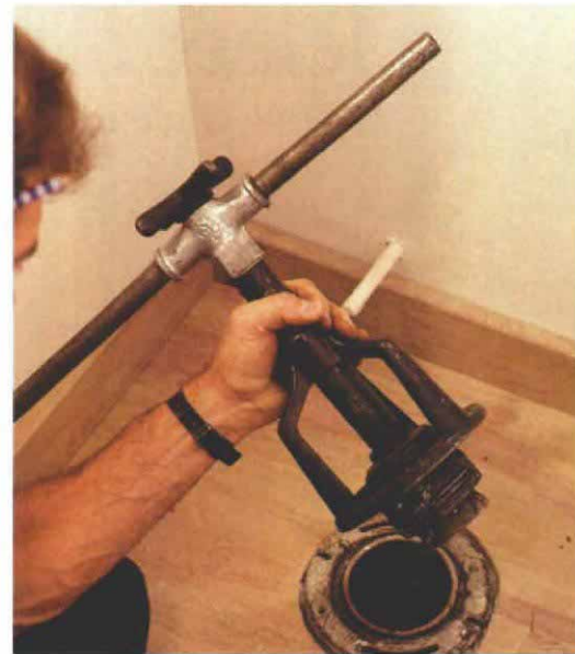
10. An internal pipe cutter will quickly trim a cast-iron stub to the desired length.
