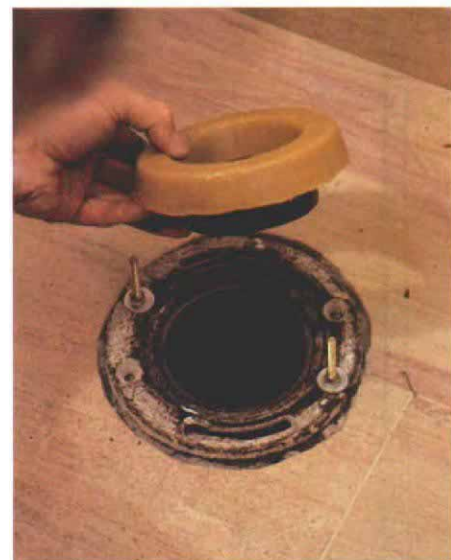
11. The transition between the toilet outlet and the closet flange is made with a wax and plastic gasket.
