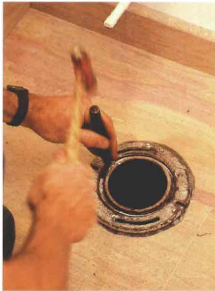
9. The hardened ring of lead is packed into the joint with a caulking iron.
